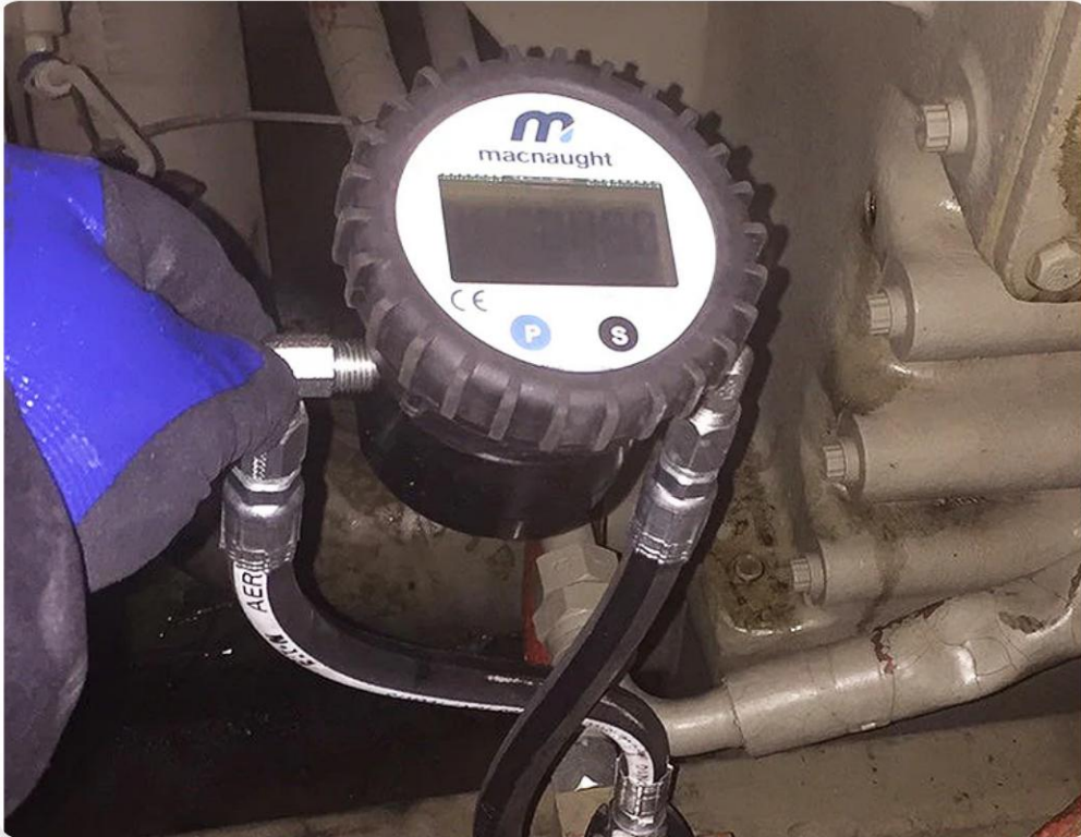
High-accuracy Macnaught flow meter, installed inline on an engine fuel line.
